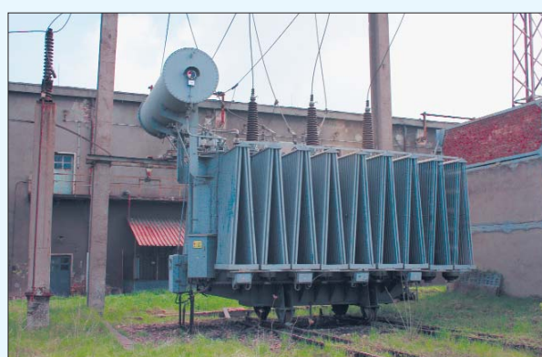
110 KV outdoor distribution installation and all commutation devices – 110 KV switches, circuit breakers.
